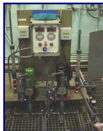
Photo 5: Polymer Feed System at Ozone Building
