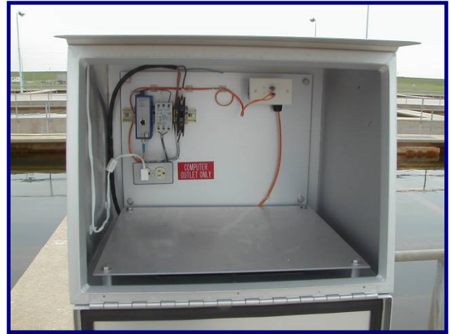
Photo 5-4 Dual Outdoor Filter Control Workstation
