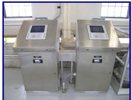
Photo 5-3 Individual Indoor Filter Control Panel with OIT
