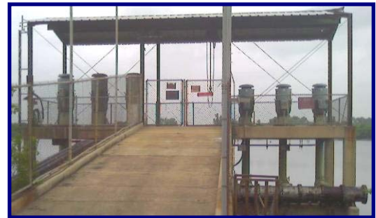
Photo 1 – Reservoir Pump Station
