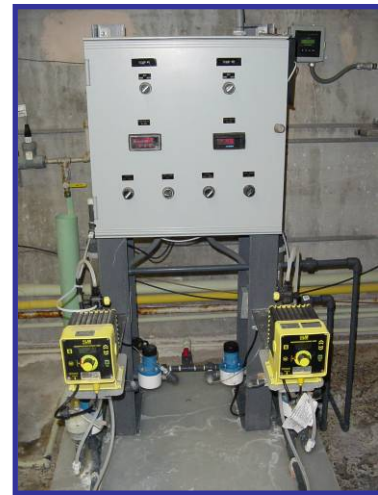
Photo 8: Zinc Orthophosphate Feed Equipment
