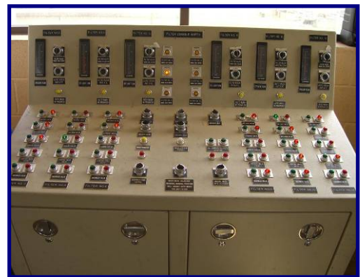
Photo 5-2 Dual Indoor Filter Control Panel
