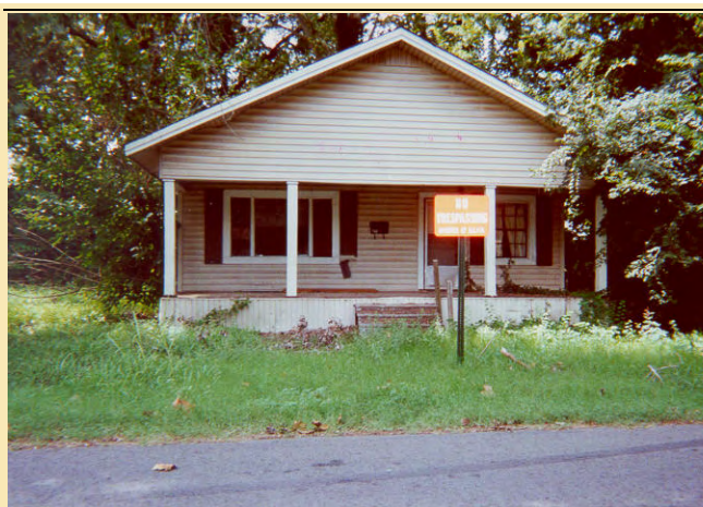
Timely and steady attention to identification, mitigation and/or removal of unsafe and dilapidated structures is needed to avoid general decline in neighborhoods at risk of losing their stability.
