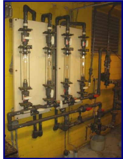
Photo 7: Chlorine Feed Equipment
