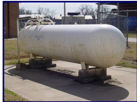
Photo 6: Ammonia Storage Tank
