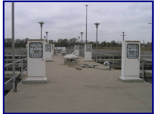
Photo 5-1 Individual Outdoor Filter Control Panel
