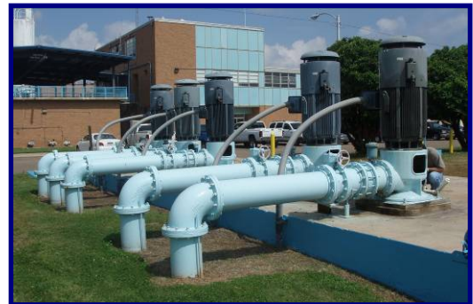
Photo 4: High Service Pump Station No. 1
