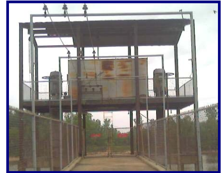
Photo 2: North River Pump Station
